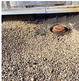
Roof Drain Flashing Leaks into Gymnasium
