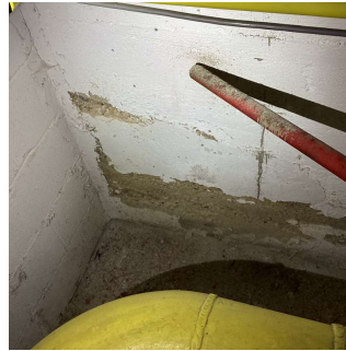
Gas Meter Room (Boiler Room, Basement Storage Area similar)
