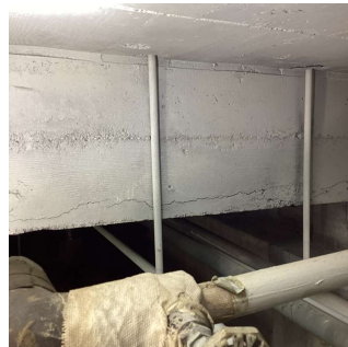
East Crawl Space (West Crawl Space, Boiler Room, Basement Corridor, Basement Fan Area, Basement Tile Storage Room similar)
