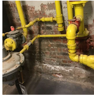
Gas Meter Room
