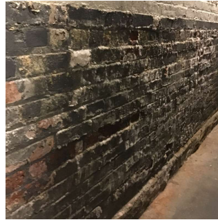
Oil Tank Room
