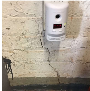
Basement (Original Building) - Fan Room
