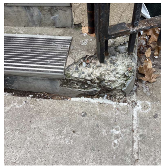
Facade M - Exit 10 No violations recorded.
