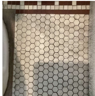
Room 411A No violations recorded.
