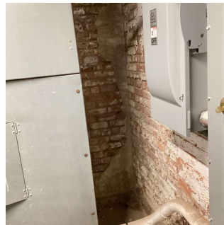
Cellar - Electrical Panel Room
