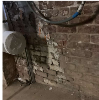
Cellar Boiler Room
