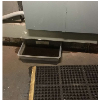
Electrical Panel Room
