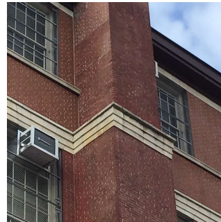
Chimney 1 Leak at Auditorium No violations recorded.
