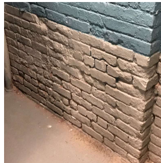
Basement Mechanical Equipment Room
