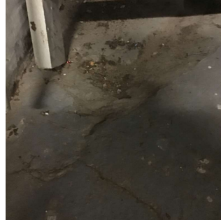
Mechanical Equipment Room Vault
