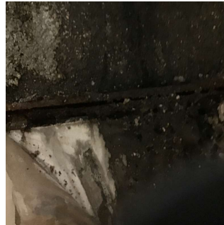
Elev Machine Room
