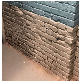
Basement Oil Tank Room
