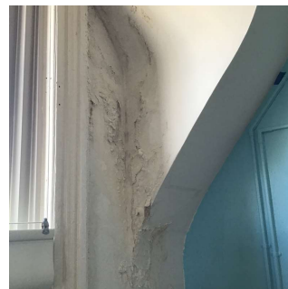
Room 401 Leak from Roof 3 Dormer
