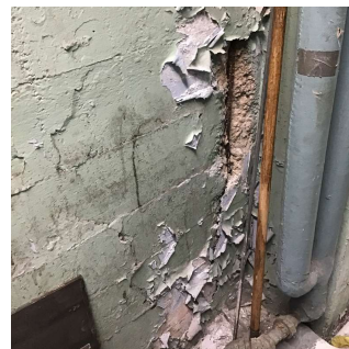
Boiler Room - Near Exit
