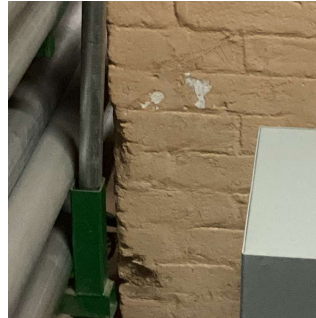
Boiler Room (Basement Fan Room similar)
