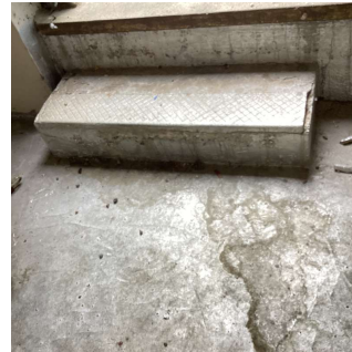
Bulkhead 1 - Damaged Step
