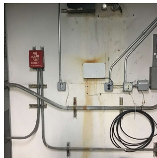
Basement - Electrical Room C18
