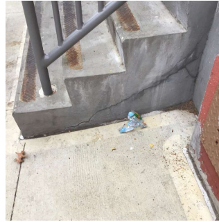
Exit 3 No violations recorded.
