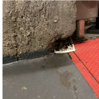
Basement - Boiler Room
