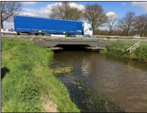
Figure 12: Bridge over a stream along the A58 between Tilburg and Eindhoven. This is one of 11 stream crossings in the InnovA58 project (Source: FHWA).
