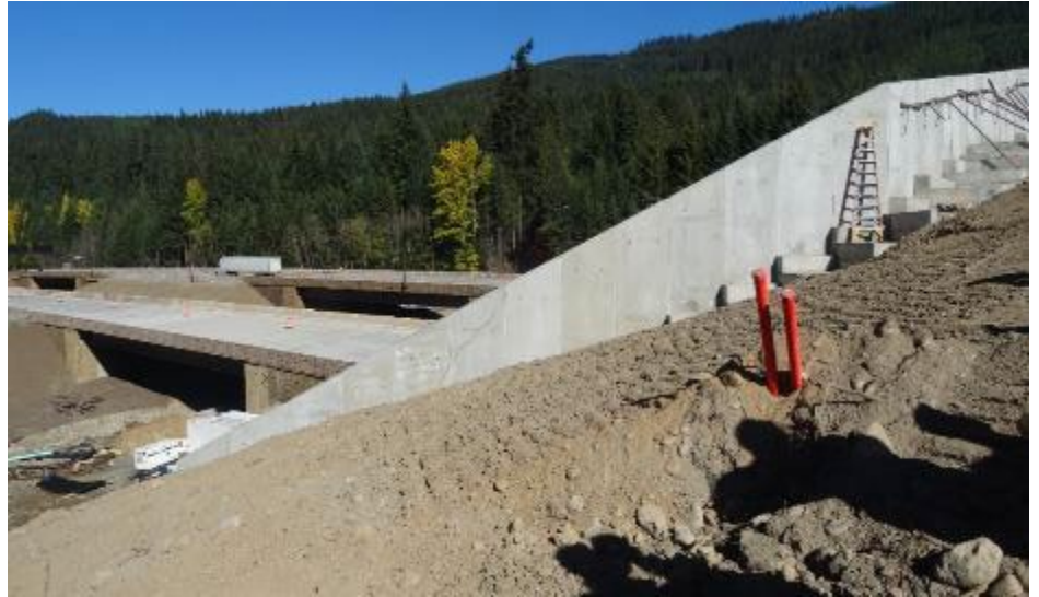
Figure 29: The project team visited a habitat crossing under construction on Interstate 90 near Snoqualmie, Washington. (Source: Volpe Center).
