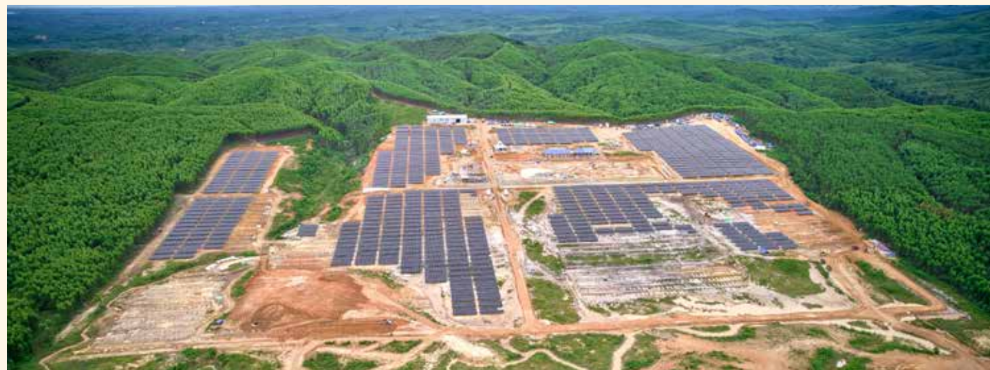
A total of 21,600 solar panels have been installed at Nusantara Solar Power Plant.
