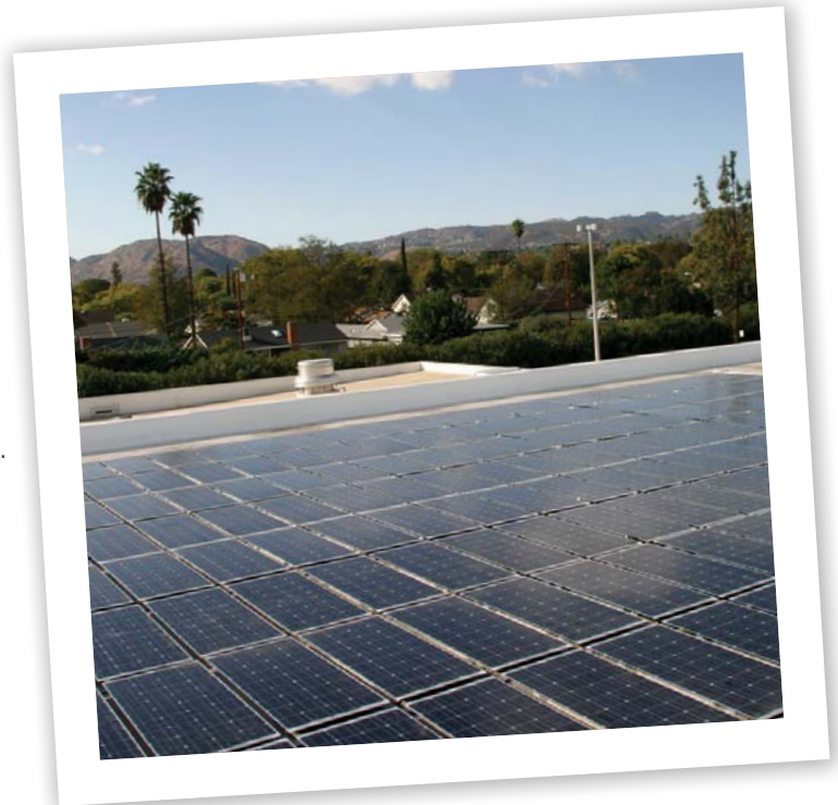
Solar roof panels harness the sun’s energy at a Los Angeles Target store.
