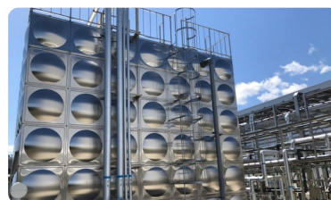
Water treatment facilities at Nasu factory (Japan)
